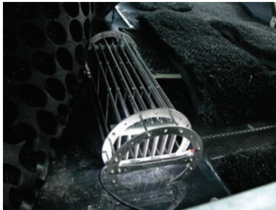
Fig. 4. MOLLIK-module installed at cooling basin (Körner et al., 2015)
