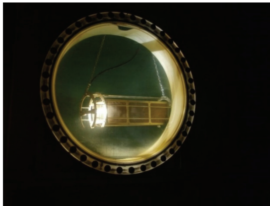
Fig. 6. MOLLIK-module installed at storage water tank of whirlpool
