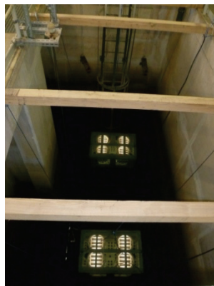
Fig. 9. MOLLIK-module at make-up supply of power plant
